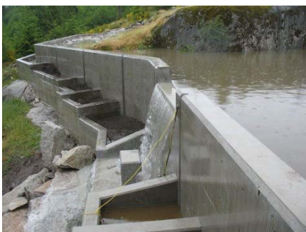
Detention Pond Outlet, Sechtel
