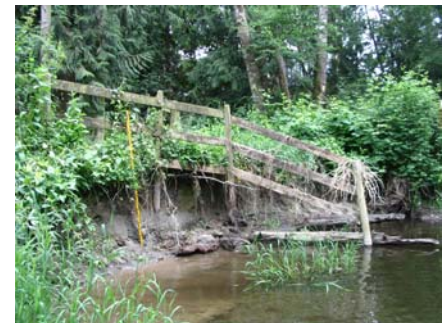
Streambank scouring along Little Campbell River in Surrey, BC
