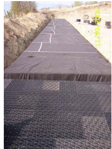
An infiltration gallery during installation at Turtle Mountain in the City of Vernon, BC.
