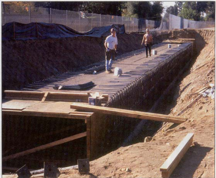
Crews work on the 3.0-meter-wide x 1.5-meter box culvert, which is large enough to take a 100-year rain event.
